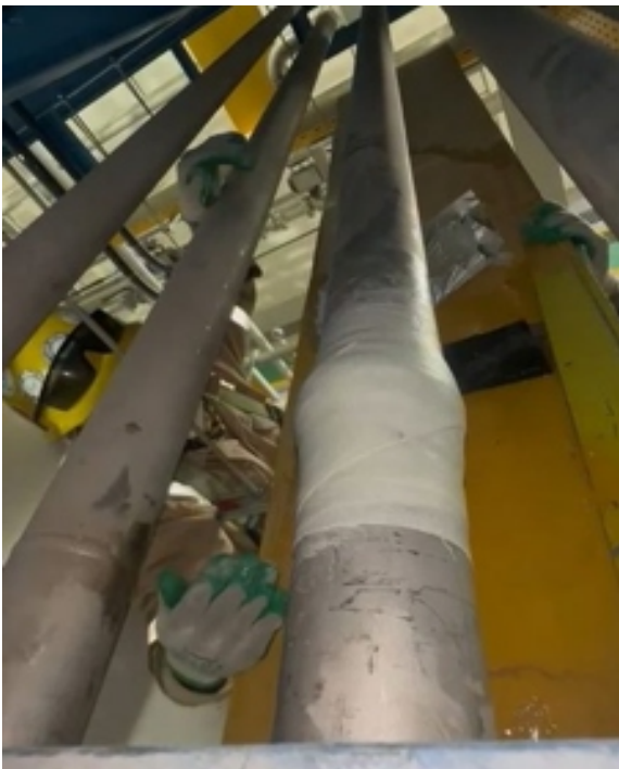
The repair was reinforced by using SylWrap HD to create a rock-hard shell around the pipe
