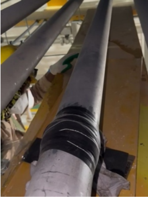
Wrap & Seal amalgamated to form a solid rubber band which contained the 3 bar methanol leak
