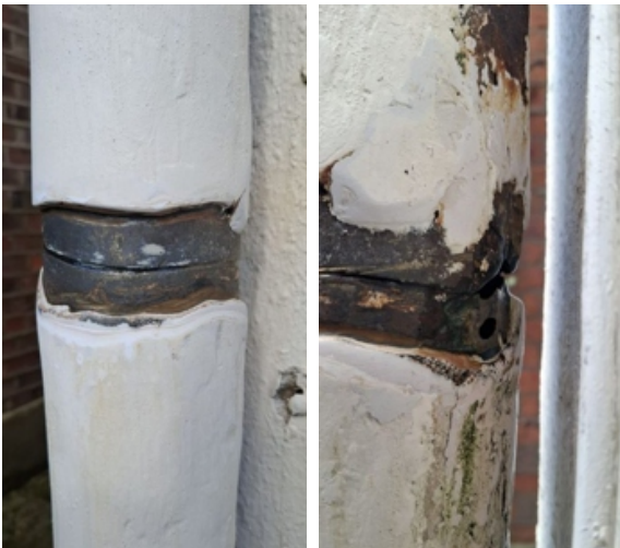
A previous failed repair attempt was ground away, creating a large groove around the crack which could be more easily filled with AB Original
