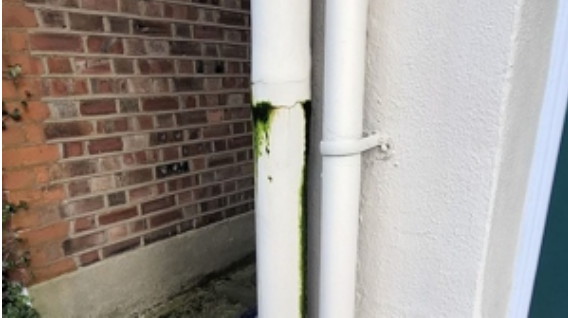
The soil pipe was leaking through an unsightly crack right next to a door into the house
