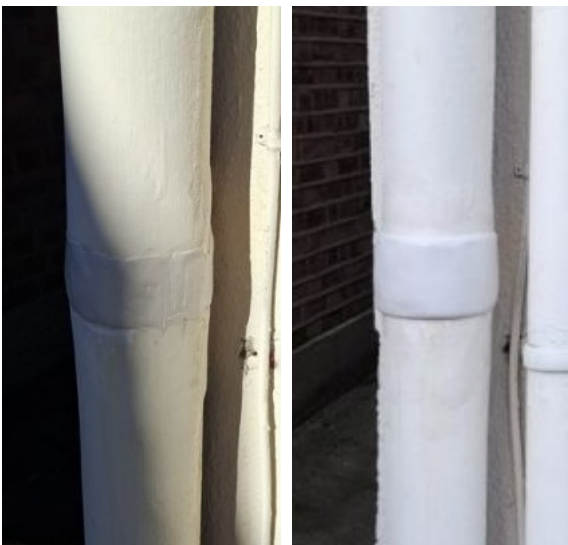
After the crack was filled, AB Original was formed into a band and bonded over the repair area to disguise it by resembling a step joint
