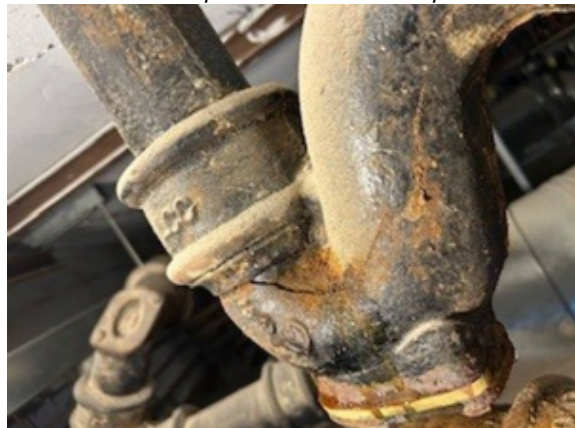
A hairline crack was found in the cast iron U-bend, through which wastewater was leaking
