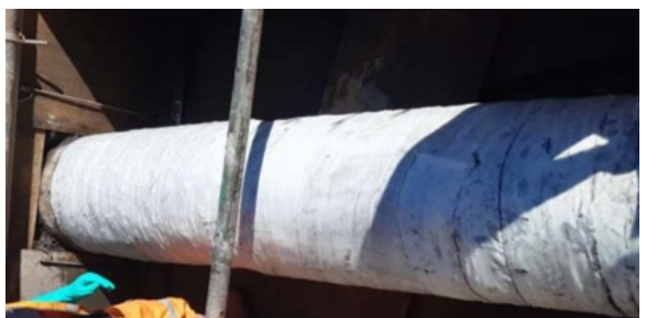
SylWrap HD was wrapped across the entire length of the pipe, completing the repair
