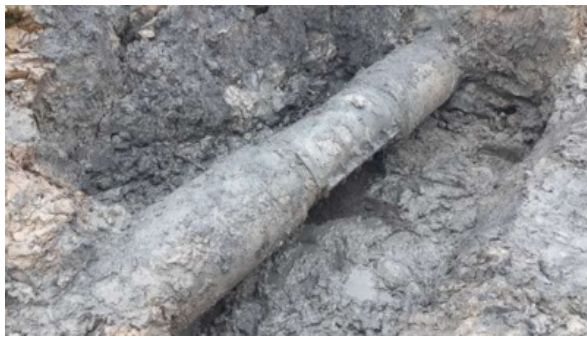
The leaking section ran beneath salt marshes, leaving an eight hour window whilst the tide was out to access, excavate and clean the pipe, and seal the leak
