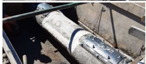
AB Original encapsulated the clamp, sealing all areas which the pipe was leaking from
