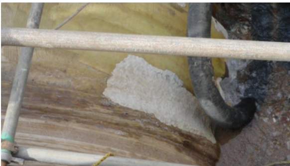
Sylmasta AB Original was used for larger leak areas because of its longer work time
