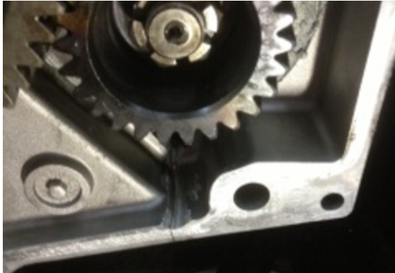
The hairline crack in centre of the metal casing
