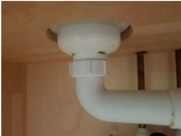
Cracks had appeared in the top of the PVC plastic drain pipe where it connected to the sink
