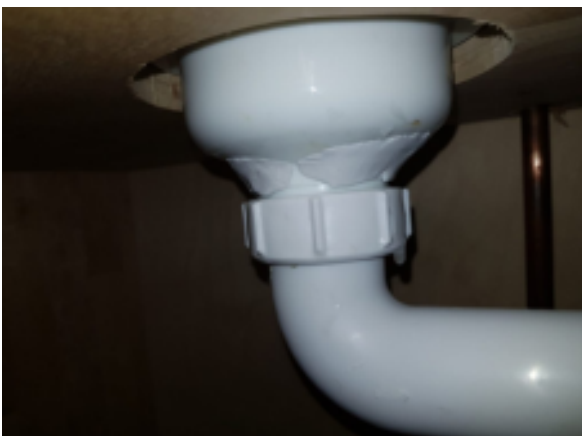
The putty hardened, permanently sealing the cracks in the pipe and preventing any more water from escaping when the sink drained
