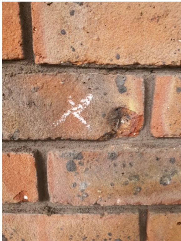
Damaged caused by lime blow can be seen next to the 'X' marked in the brickwork
