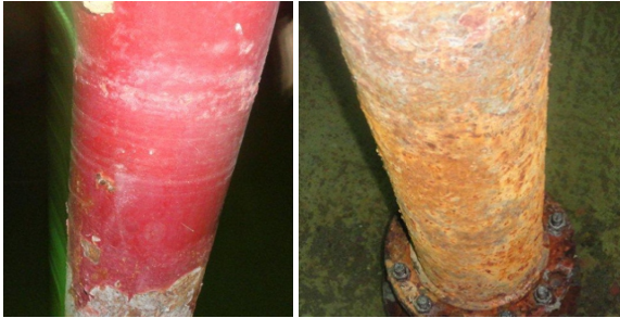
The steel pipe was badly corroded, especially in its lower sections beneath the surface of the reservoir
