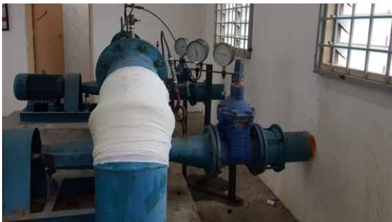
Repairing the elbow was completed in less than 30 minutes with no disruption to operations at the pumping house or local water supplies
