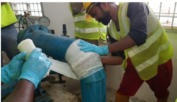
SylWrap HD reinforced the initial repair by creating a rock-hard, impact resistant sleeve around the pipe
