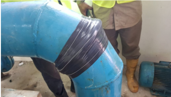
Wrap & Seal was stretched by 300 percent as it was wrapped around the pipe, amalgamating to itself to form a solid rubber band containing the 6 bar leak
