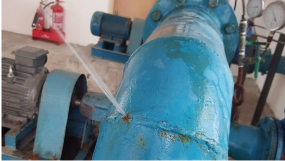
A pressurised jet of water was escaping the elbow bend at 6 bar through a pinhole left by corrosion
