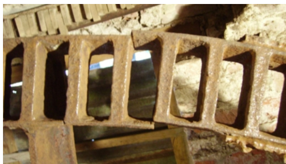
Damage caused to the original cast iron castings
