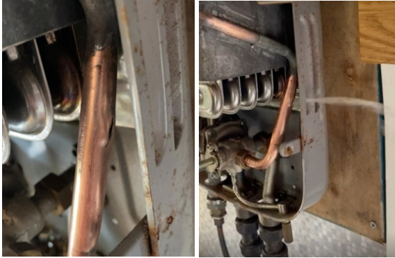
The crack in the copper pipe was difficult to access. Whenever the boiler system was turned off, a jet of pressurised water sprayed from the hole
