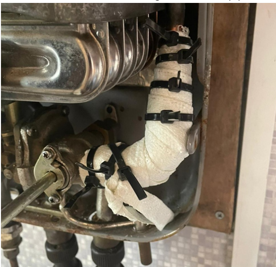
The space constraints meant SylWrap HD was cable tied in place whilst it cured, reinforcing the repair with a rock hard, protective outer shell
