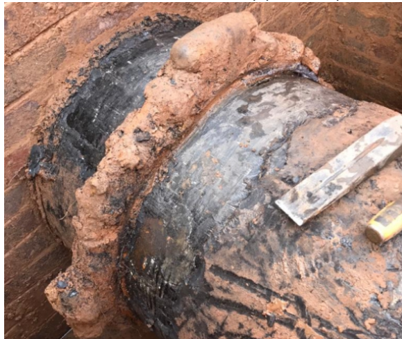
Raised couplings created a difficult ridge shape to seal
