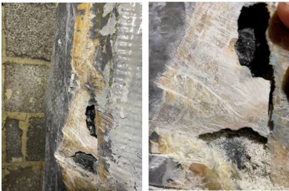
Water was leaking from two deep cavities in the pipe
